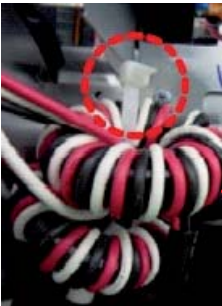
► Fix Comp Wire-Core to Bracket Beam Control Box using large size Cable Tie(350mm).
